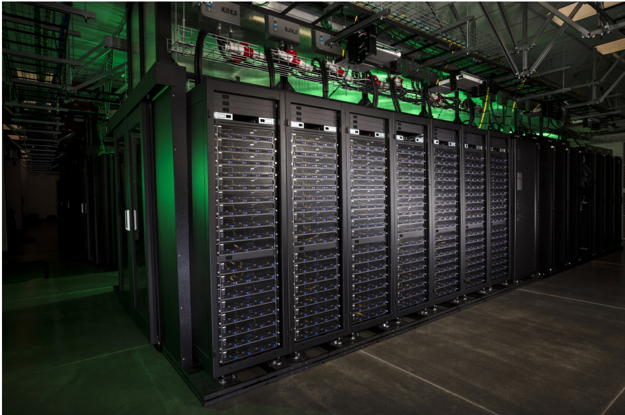
Figure 2-3. Sandia's Glinda HPDA Platform
